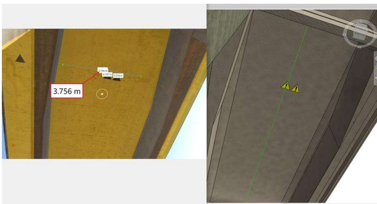
Figure 13. Efflorescence and crack measurements at the bridge slab.
