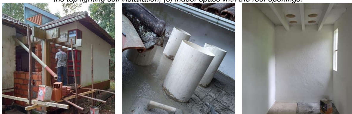
Figure 1: (a) Building chamber for performance monitoring under construction; (b) roof openings for the top lighting cell installation; (c) indoor space with the roof openings.
