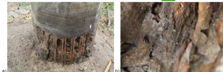
Figure 5. Main damage to the bridge; Severe corrosion on pillar 01 (face 2).
