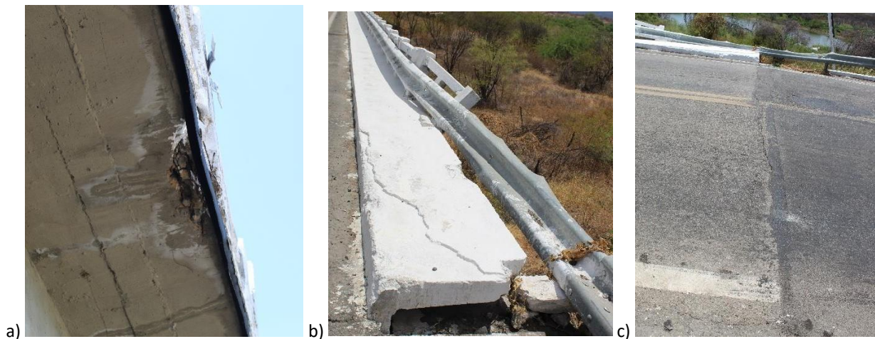
Figure 10 – Unrepaired damage: a) Damage to the right flange of the slab; b) Damage to the reinforced concrete guardrail; c) Damage to the asphalt pavement due to missing or inadequate expansion joint
