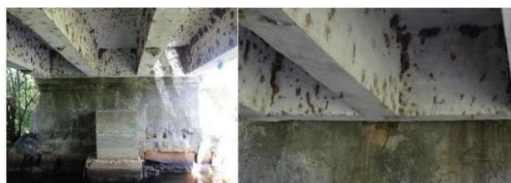
Figure 2. Bridge 140132: (a) abutment 2; (b) dump spots and biological degradation.
