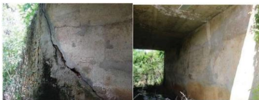
Figure 12. Bridge 140136: (a) a large diagonal slit of abutment 01; (b) excessive deformation and deep cracks.
