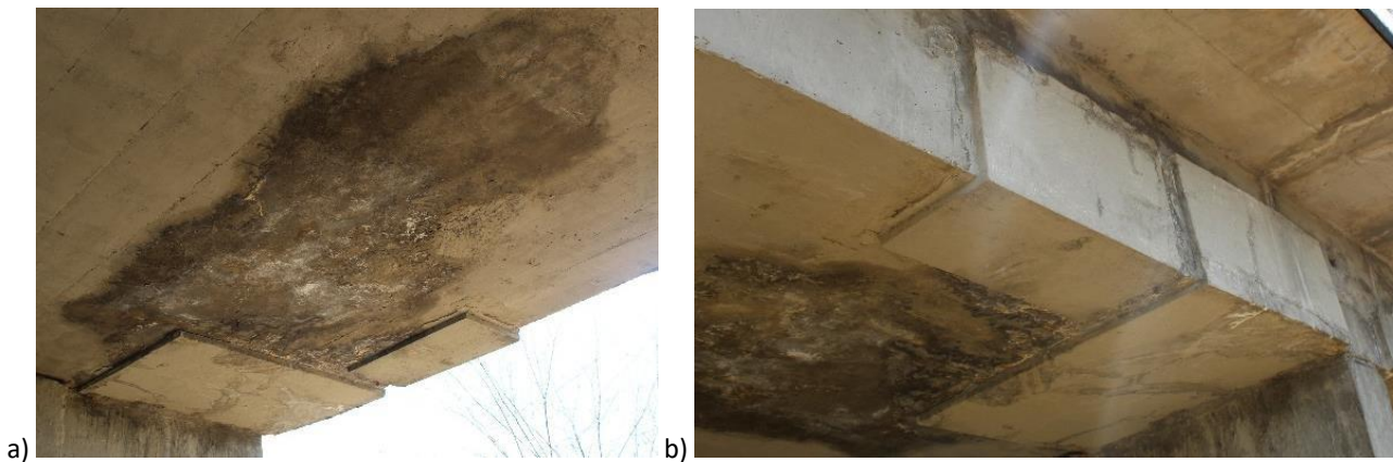
Figure 12 – Recurring repair damage due to insufficient drainage and concrete infiltration
