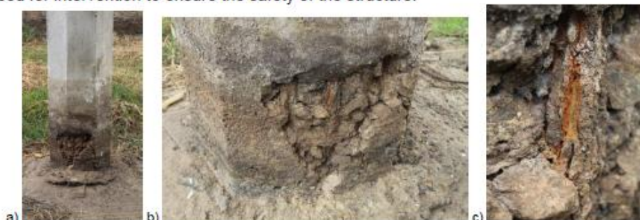
Figure 4. Main damage to the bridge; Severe corrosion on pillar 01 (face 1).
