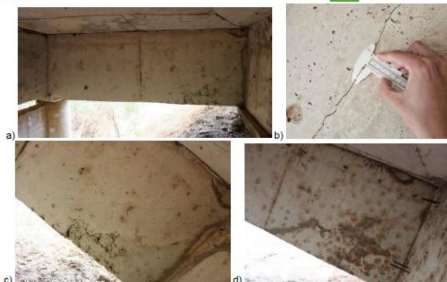
Figure 9. Main damage to the bridge; Severe cracks on beam 02.
