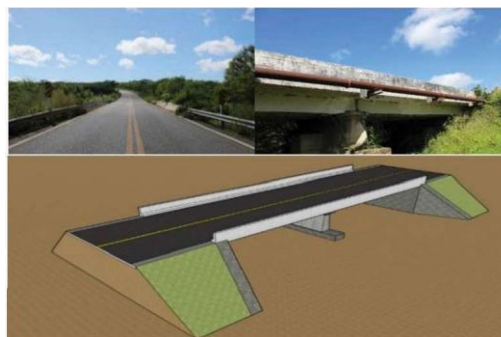
Figure 1. Km 127 bridge: (a) view of the pavement; (b) lateral view; (c) Sketchup 3D model.
