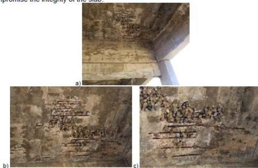
Figure 7. Main damage to the bridge; Severe corrosion on slab 02.
