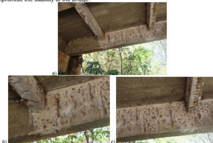
Figure 2. Main damage to the bridge; Severe corrosion on beam 02.
