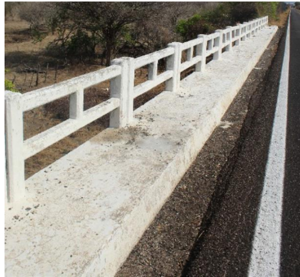
Figure 5 - Example of the type of barrier used on bridges constructed between 1960 and 1975.
