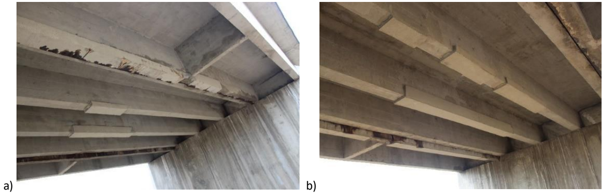
Figure 3 – Repairs to reinforced concrete beams; a) View of the 1st span; b) View of the 2nd span
