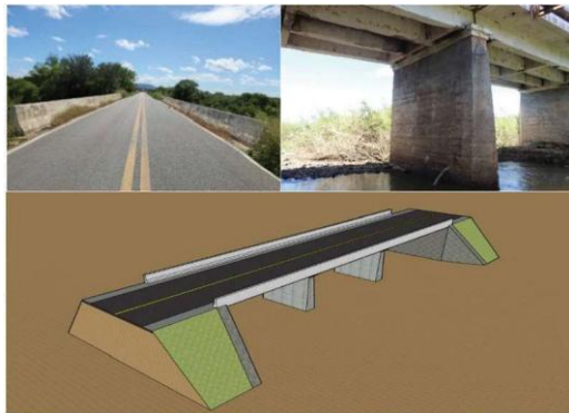
Figure 6. "Cabelo" bridge: (a) view of the pavement; (b) lateral view; (c) Sketchup 3D model.
