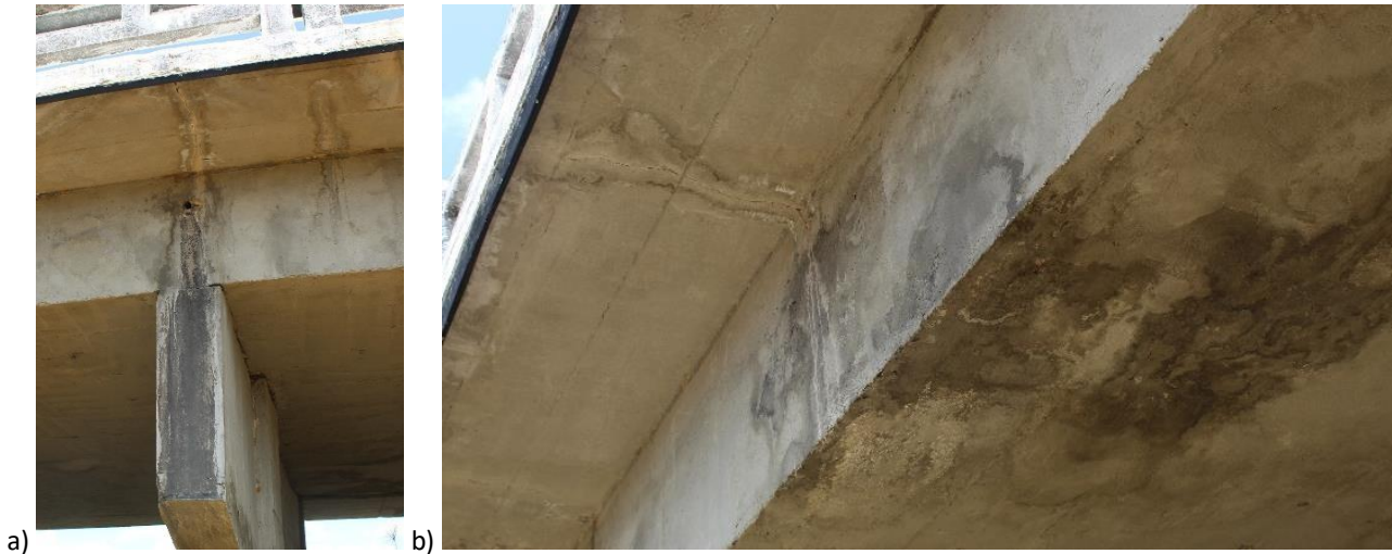
Figure 11 – Drainage deficiencies on the bridge causing recurrence of damage; a) Side hole for insufficient drainage; b) Crack in the side flange of the bridge causing infiltration
