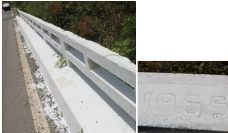
Figure 2 - Example of the type of barrier used on bridges constructed between 1950 and 1960.
