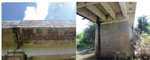
Figure 7. Bridge 140134: (a) spalling and corrosion of rebars; (b) dump spots and biological degradation.
