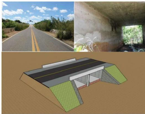
Figure 11. “Catolezinho” bridge: (a) view of the pavement; (b) lateral view; (c) Sketchup 3D model.
