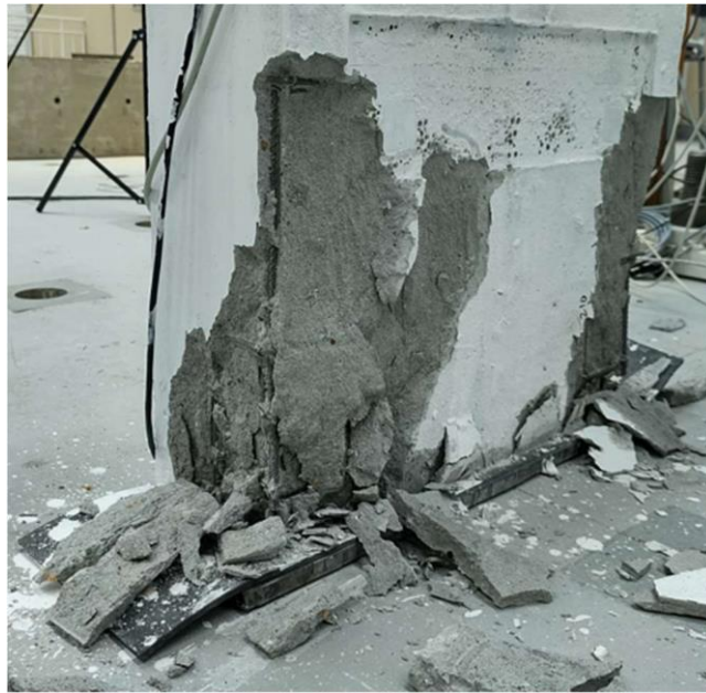
Figure 3.10 - PA5 sandwich panel failure due to stress concentration at the bottom end.
