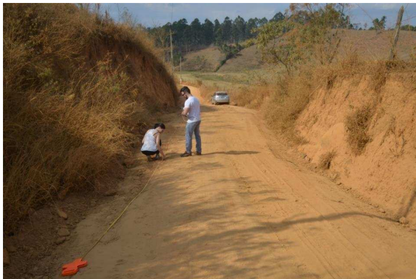
Figure 1: County road from Minas Gerais (Brazil) in poor condition.
