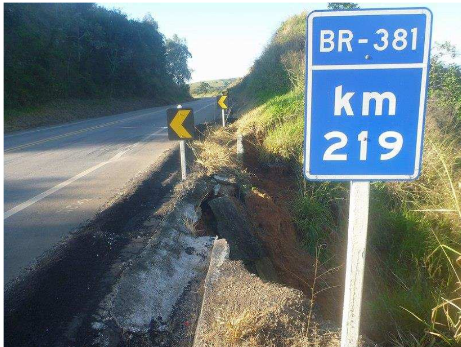
Figure 1: Paved road from Minas Gerais in poor condition (CNT, 2018).
